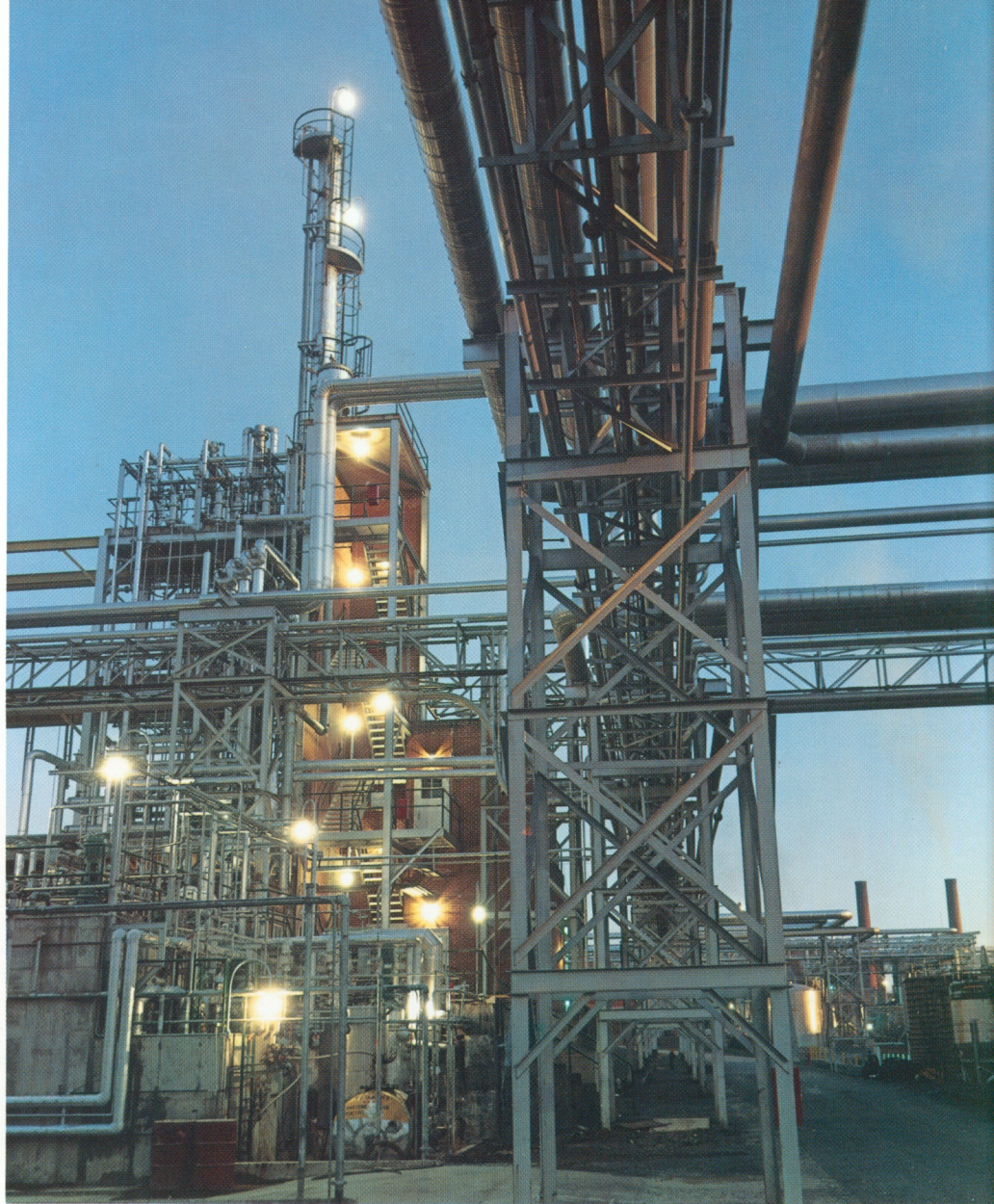
A distillation column at Tennessee Eastman Company, Kingsport, Tennessee
